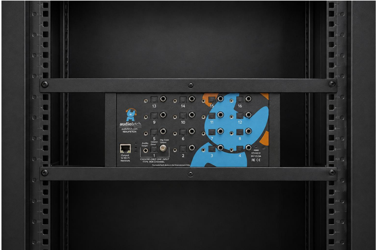
Installed AudioFetch unit shown in a standard 19-inch equipment rack.
